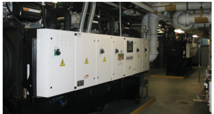
450-ton Smardt chiller featuring 5 Danfoss Turbocor compressors
